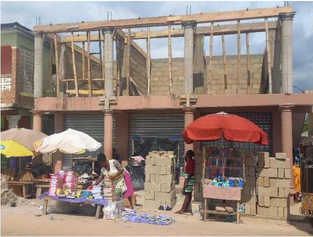
1 No. 3 Unit Trading Store at Asikuma Market Ph.II lintel level completed (Opposite GOIL) IGF
